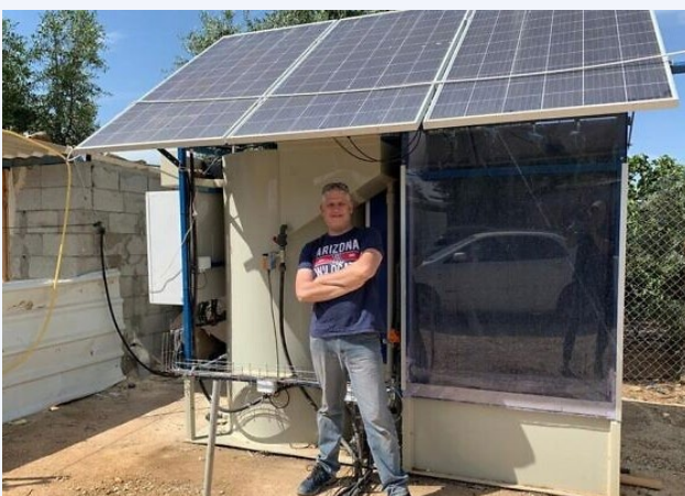
Off-grid wastewater treatment plants (WWTP)*
